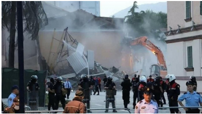
Demolishing of the National Theater Tirana May 17, 2020. Photo taken by : Nikola Đorđević, Emerging Europe.
