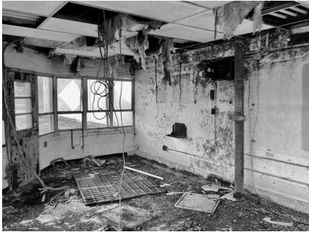
Interior of SAGE blockhouse that has come to disrepair, Stewart International Airport- Newburgh, New York
